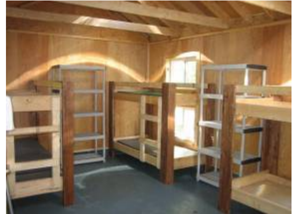
The interior of the new "Beaufort" camper cabin. Work continues on the new Shower House, and the kitchen renovation of the Dining Hall.
