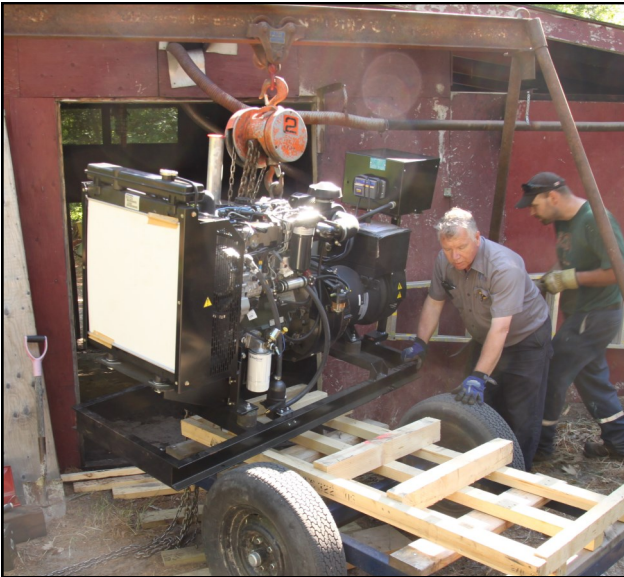
Generators do not last forever. In this Jody Waddell and electrician Don Harrison move a new generator into the Gen Shed in 2012.
