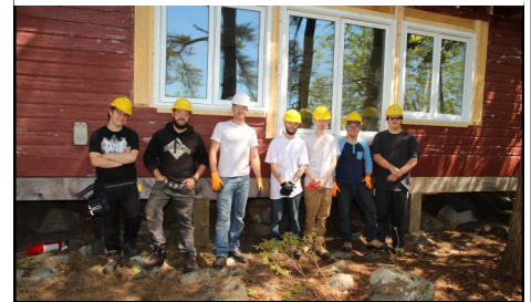
Pictured from top to bottom, - Putting the new steel roof on the cabin - The inside with new windows and a great view of the beach - The students from Lasalle Secondary who worked on the project in 2016
